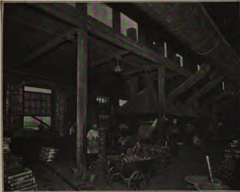
FIG. 146.—SYSTEM OF HOODS AND VENTILATORS TO CARRY OFF THE FUMES FROM THE FURNACES IN A FOUNDRY. (Mass. State Board of Health.)
